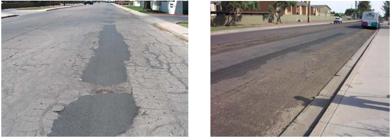
Fig. 1. (a) Pavement Condition Before the Overlay; (b) Surface Preparation by Milling off the Edge of the Pavement.
